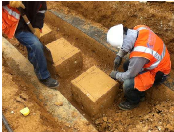
Figure 2: Extraction of undisturbed soil liner sample for in situ block density and large direct shear testing on textured geomembrane and soil liner interface
