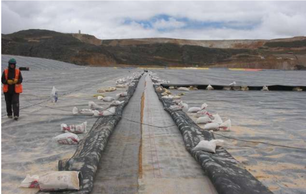
Figure 7: GCL contraction and panel separation due to insufficient overlap
